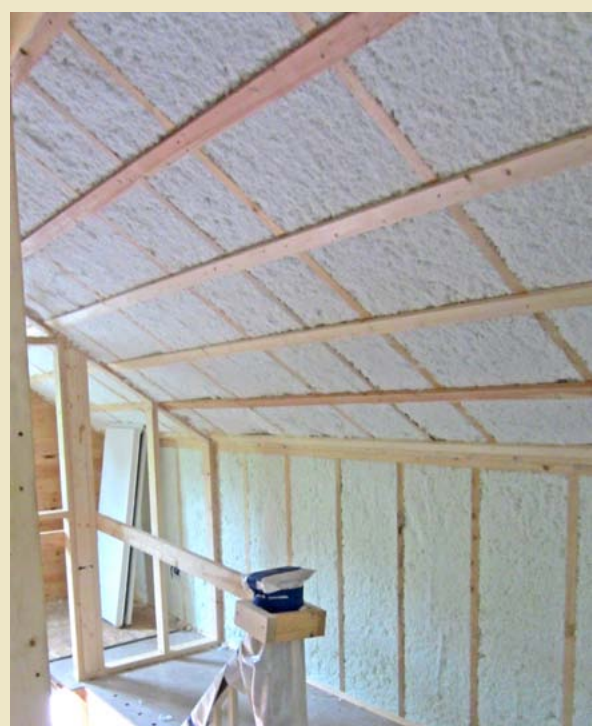
Roof / Attic: After 4" of rigid insulation was added to the roof, as well as 7" of spray fiberglass, bringing the roof assembly up to R-54
