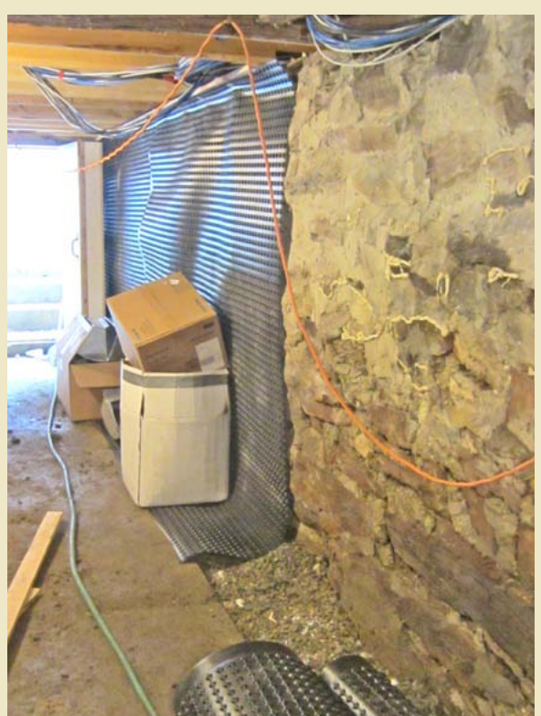
Foundation wall: After New drainage mat over the foundation wall connected to a perimeter drain trench and tied to a sump pump.
