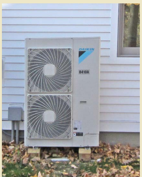
Mechanical: After Daikin ducted air source heat pump, with existing Budarus boiler gas fired backup.
