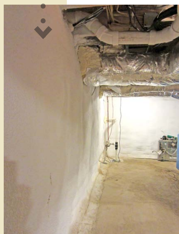
Foundation wall: After 4" spray foam insulation with intumescent paint added over the drainage mat.
