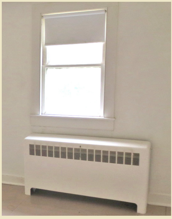
Mechanical: Before Radiators tied to oil boiler
