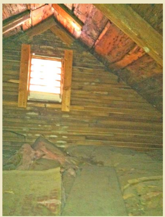
Roof / Attic: Before Minimal batt insulation in attic.
