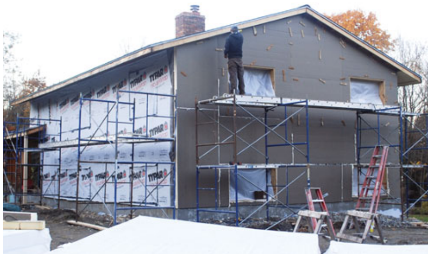
Figure 2. After removing the old windows and installing plywood window bucks, workers wrapped the walls with 4x8 panels of 4-inch-thick polyisocyanurate foam (top). The panels were glued to the vertical cedar siding, and plywood cleats secured with long screws were used to temporarily hold them in place until the glue set (center and above).
